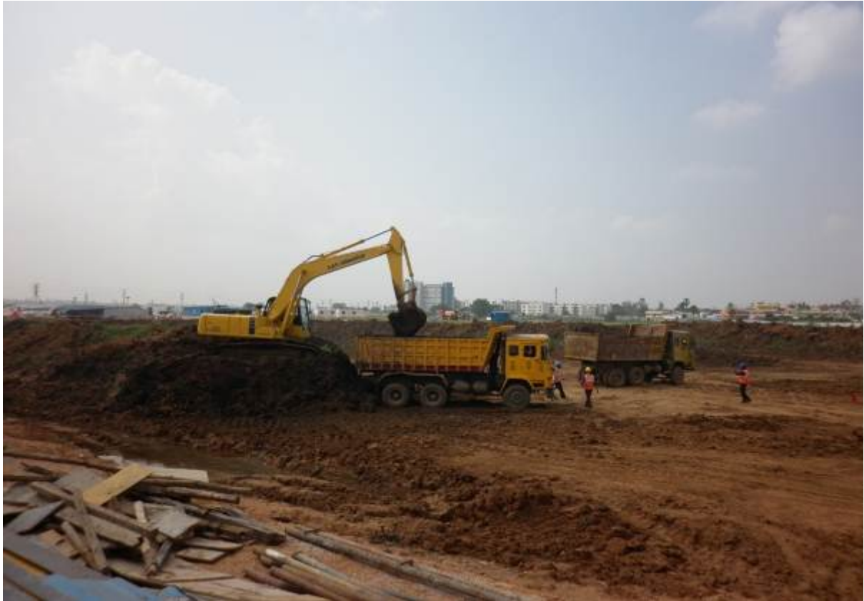
Excavation is in progress at Zone-1 Part-2 & Zone-2 Part-2 area at Nagole Depot
